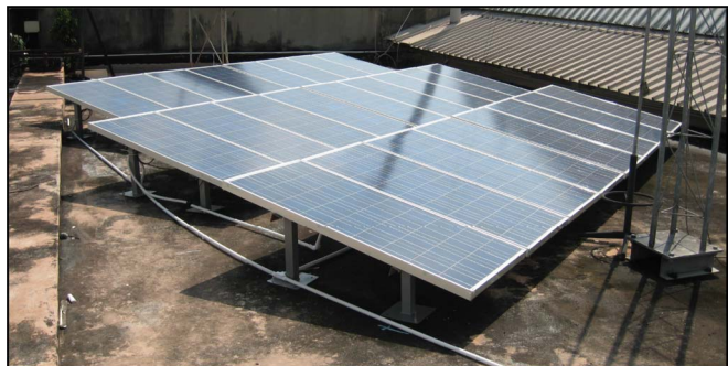
Fig. 6. Solar panels used in the experiment.
